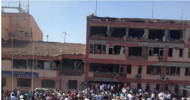
a) Building damage due to a terrorist attack targeted Elazig Police Headquarters (Aljazeera, 2022)
