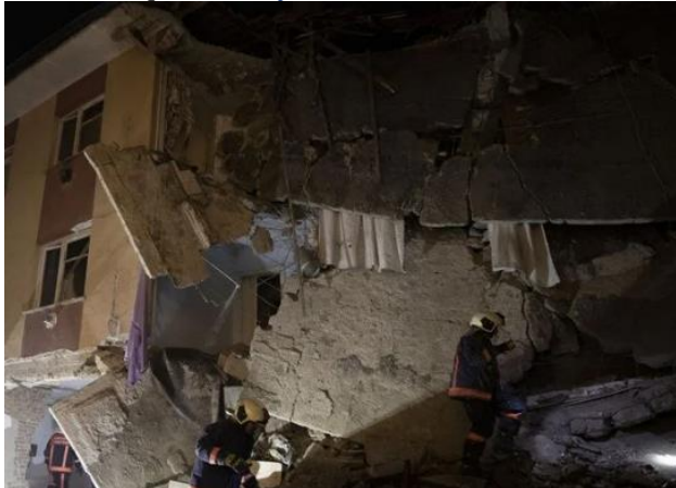
b) Structural damage due to an explosion happened on an apartment building in Ankara (NTV, 2022)
