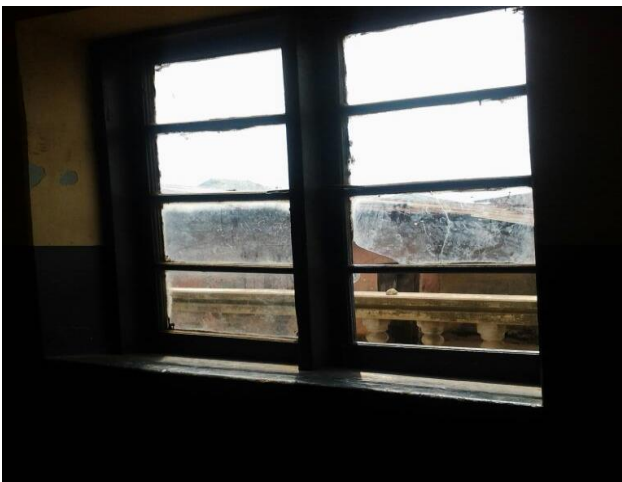
Figure 13: Broken glass window with wooden frames
